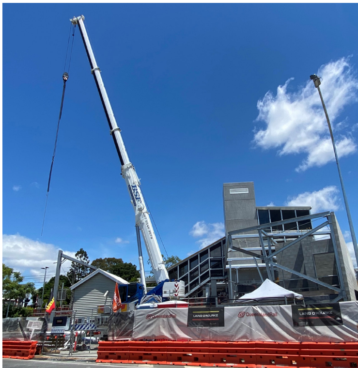
Above: Construction of the new Banyo station entrance plaza and footbridge, viewed from St. Vincent's Road.
